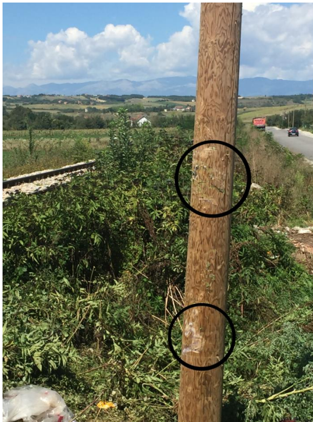
Fig. 16. The spots on the electric pole left by the vehicle after the impact (Source: RRA).
